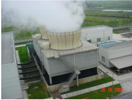
Figura 2.2 - Torre de resfriamento de tiragem mecânica (Fonte: http://www.swlf.ait.ac.th/Old/Visu_CD/photo_collection/china/fieldvisit/Cooling%20Tower%20at%20the%20Incineration%20plant.JPG ).
