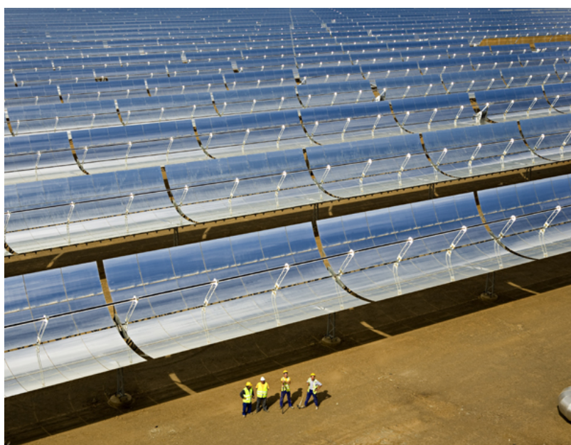
Figura 15. Central Andasol - 3 (Solar Millenium). [16]
