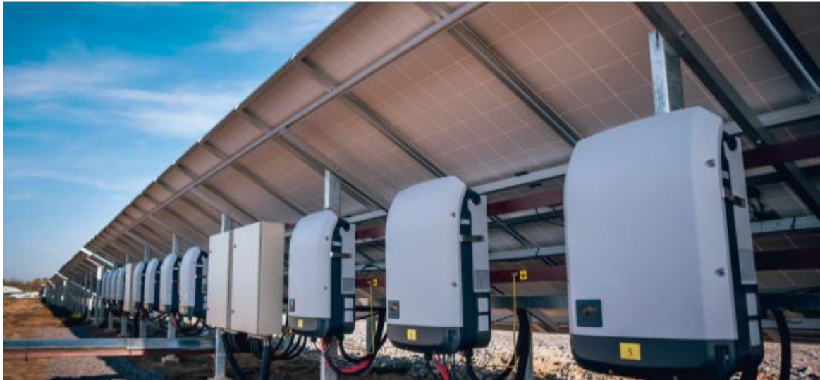
Figura 2.8: Inversores fotovoltaicos (Boreal Solar, 2021).
